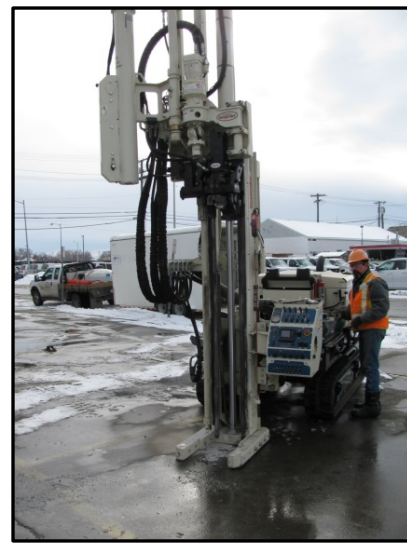
GeoProbe rig installing soil boring at a former service station, Billings (Jan. 2016)
